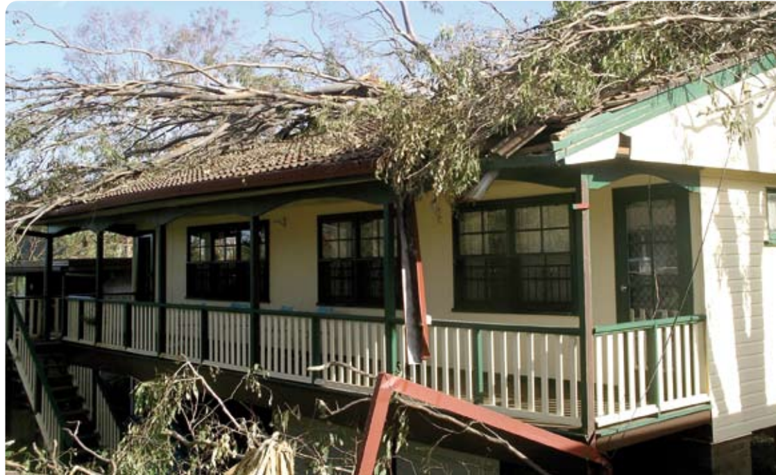
Damaged homes from the Queensland Storms, Nov 2008
